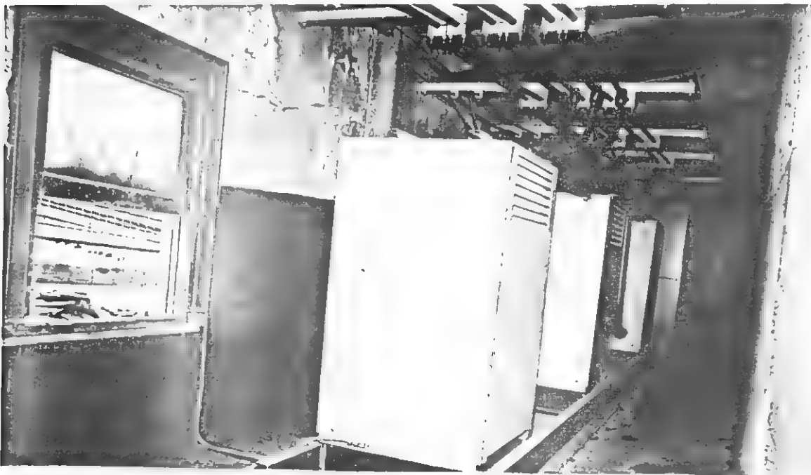
At second floor of YMCA Building, condensers line the western corridor.
